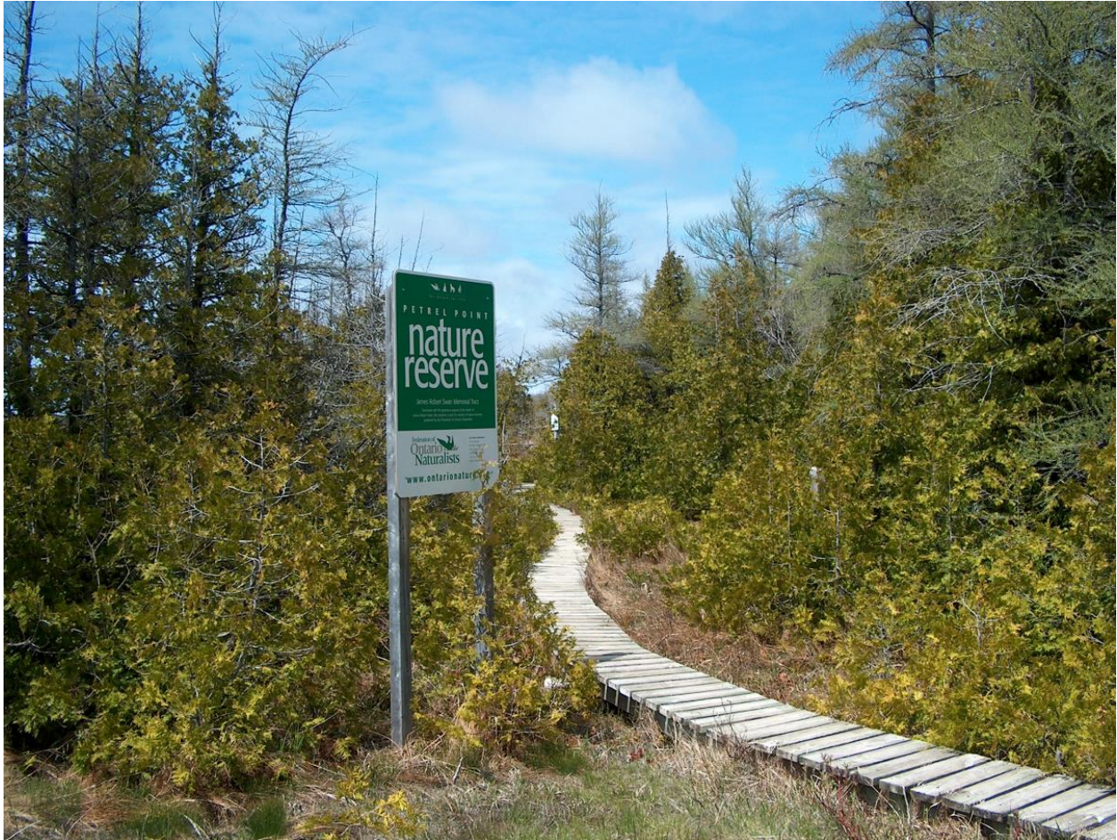
Figure 2. Boardwalk section prior to decommissioning. While the boards look to be in reasonable condition, many are detached, and the cribbing is rotten (as seen in Figure 1).
